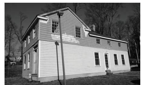
The bow window has been removed from the Levi Cory house in order to restore it to its original state.
